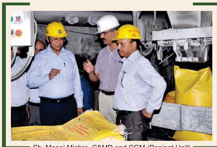
Sh. Manoj Mishra, C&MD and CGM (Panipat Unit) at the bagging section of the Plant
