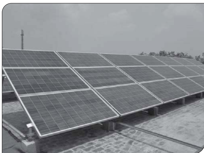
A view of solar power plant at Corporate Office, Noida
